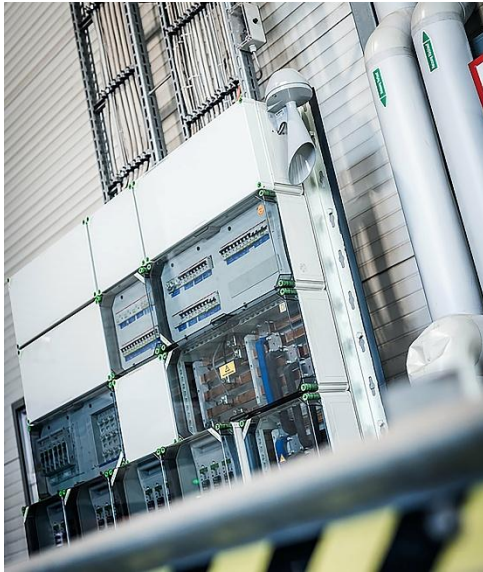
Image 3: Spelsberg's qualified employees handle everything from the initial design to the final production of electrical panels, guaranteeing perfect results
